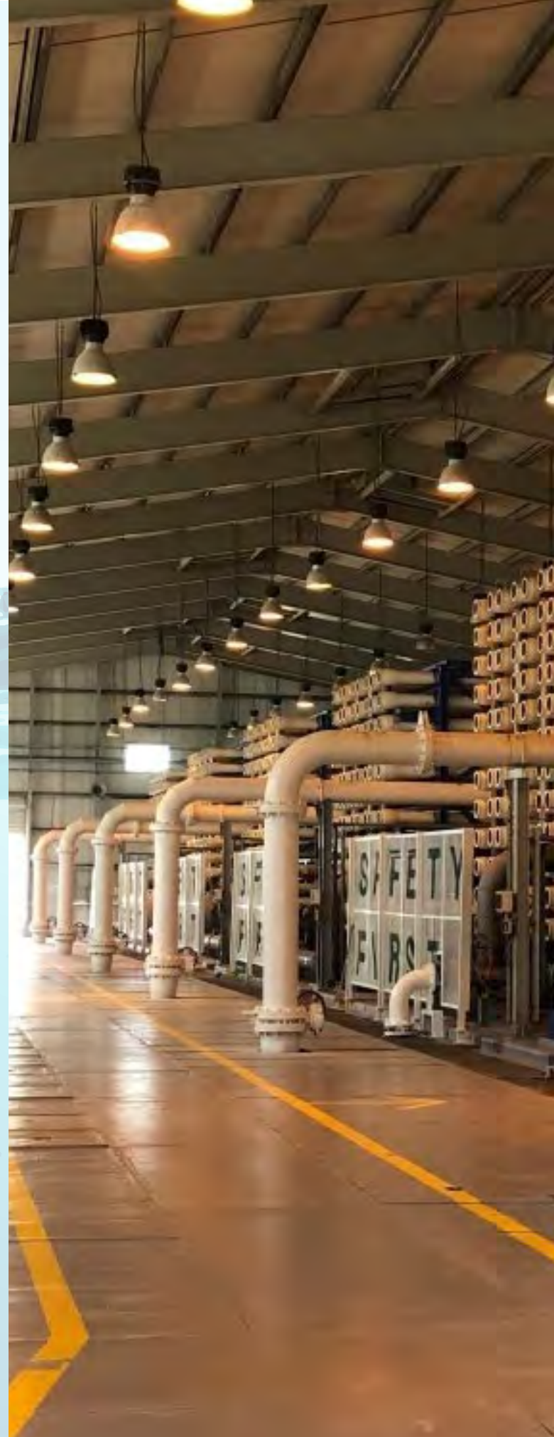
Desalination plant at King Abdulaziz International Airport in Jeddah (Saudi Arabia)
